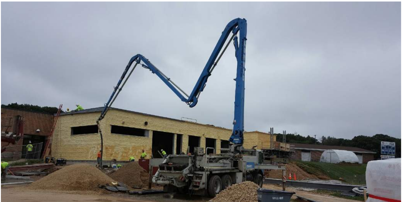
Shown above is a picture of the pump truck which is being used to pump concrete into the school. Here it is being used to help pour the slab in the new addition!
