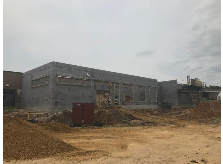
A look at the progress on the new STEM addition. CMU walls are nearly complete!
