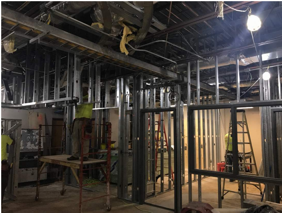
Steel stud is near completion and sits ready for the drywall to be hung.
