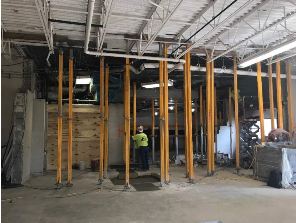
Shoring is in place to support the new opening between the weight room and tech ed. areas.
