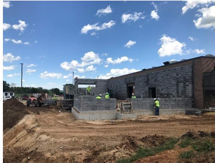
This picture shows the progress on the STEM Addition from the northwest. It provides a great view of the completed and backfilled foundation wall as well as the block being set on it! In addition to Technology Ed. space, there will also be new bathrooms and concessions area.
