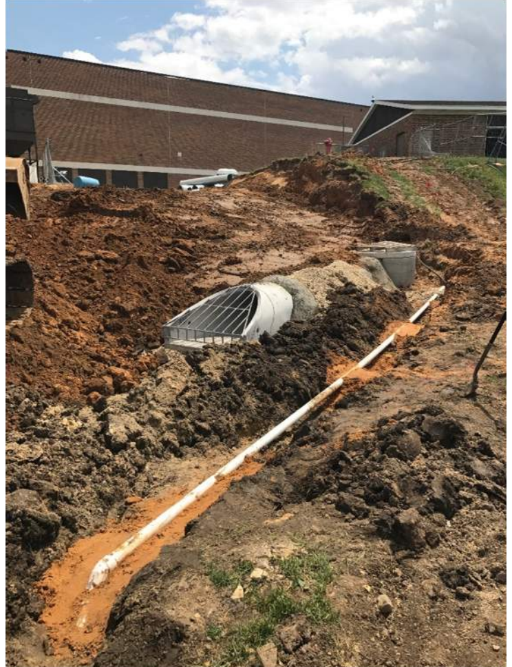
A second view of storm line that was re-routed during this weeks exterior site work
