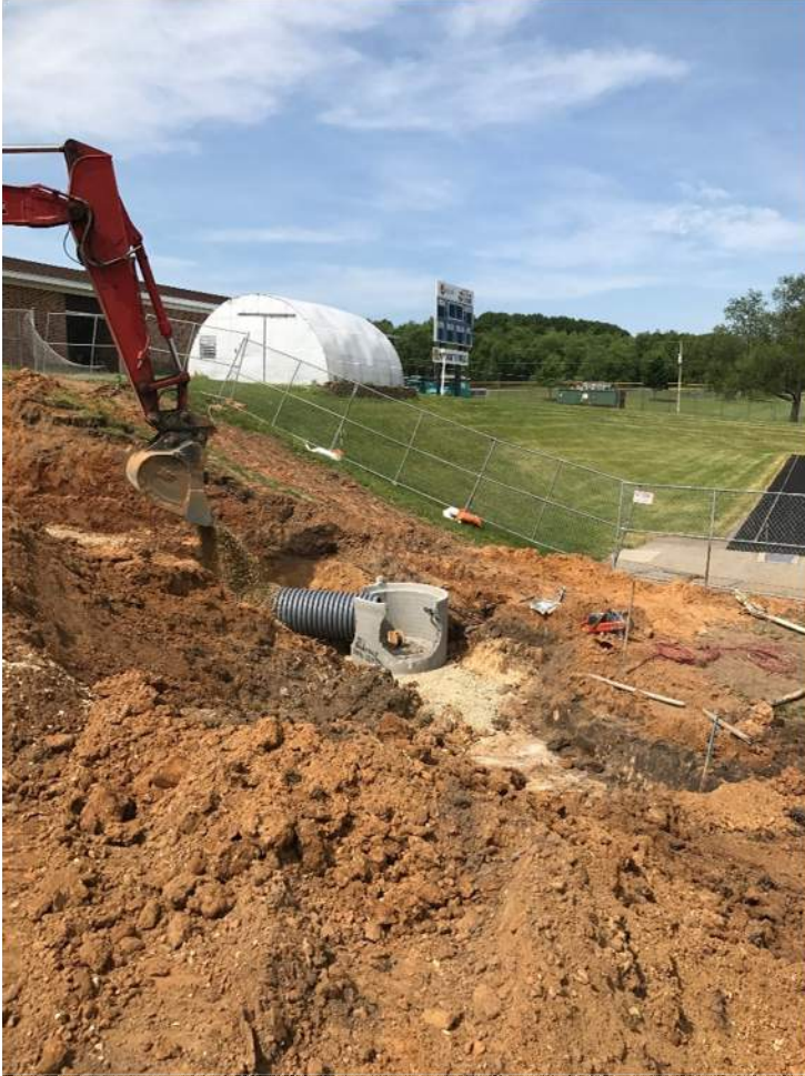
A view of the underground storm line that was re-routed around the footprint of the new addition.
