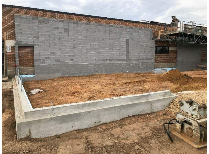
A look at the progress on the North end addition. This view shows the new CMU fire wall that will lay in between the new and existing STEM areas
