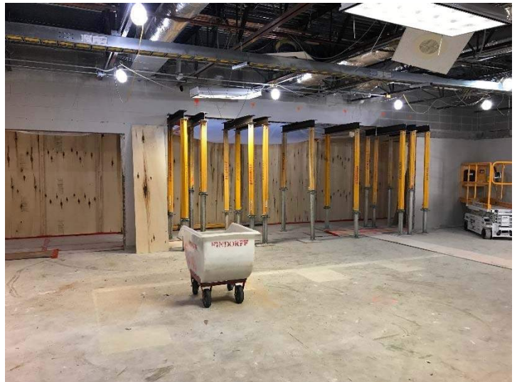
A picture showing the progress in the reception area at the High School main entrance
