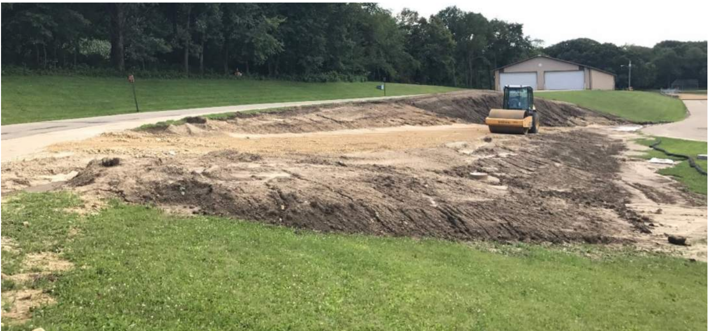
Shown above is a picture of a roller which was used to compact the newly excavated road coming off of Hayden Drive!
