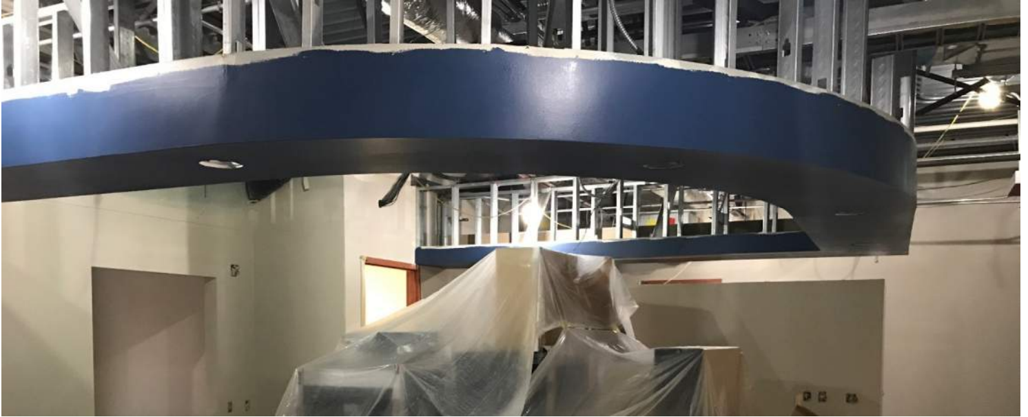
Shown here is the soffit that will fall above the new casework in the secure entry area. Look at the fresh coat!
